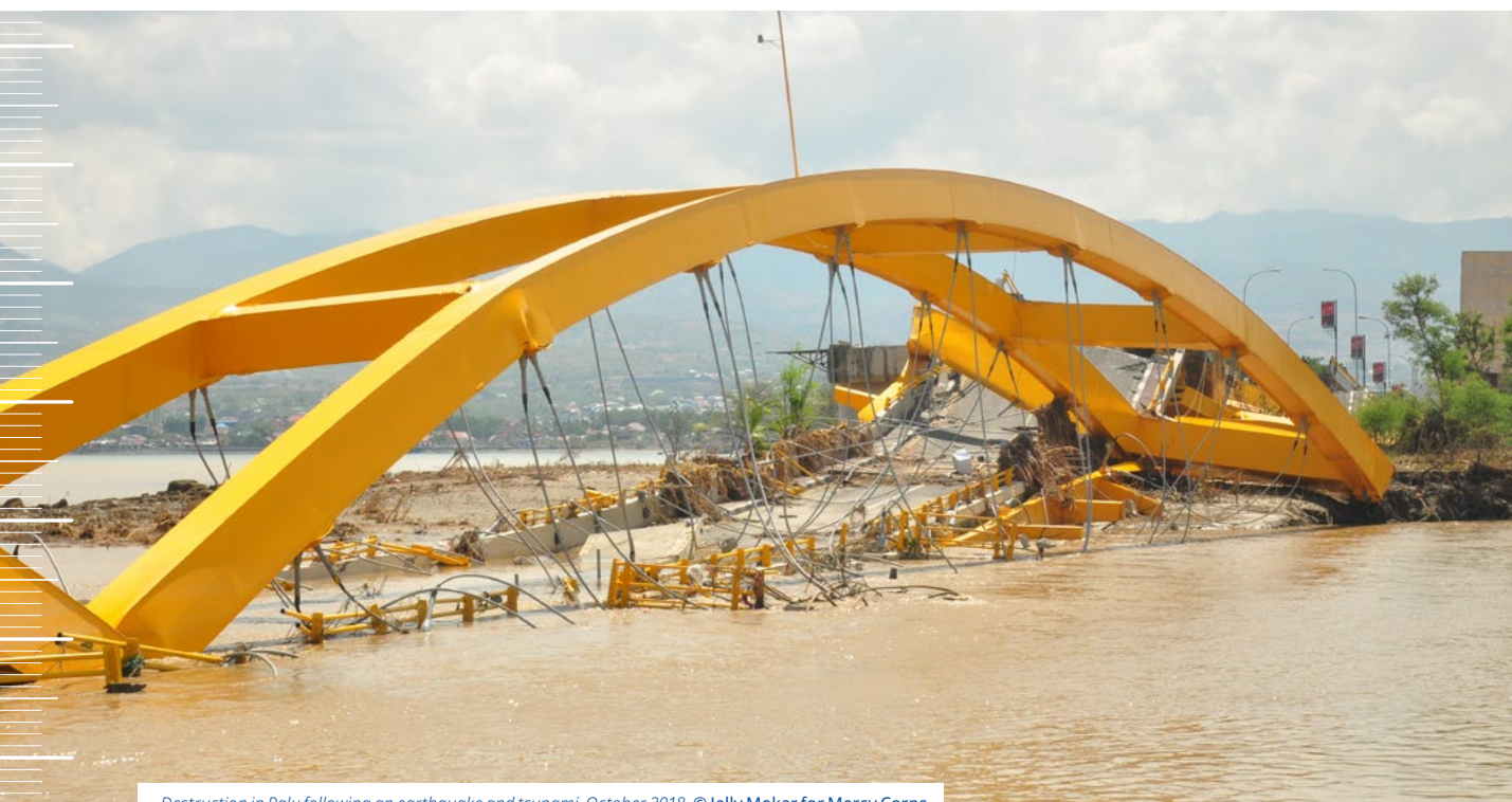
Destruction in Palu following an earthquake and tsunami, October 2018. © Jelly Mokar for Mercy Corps
