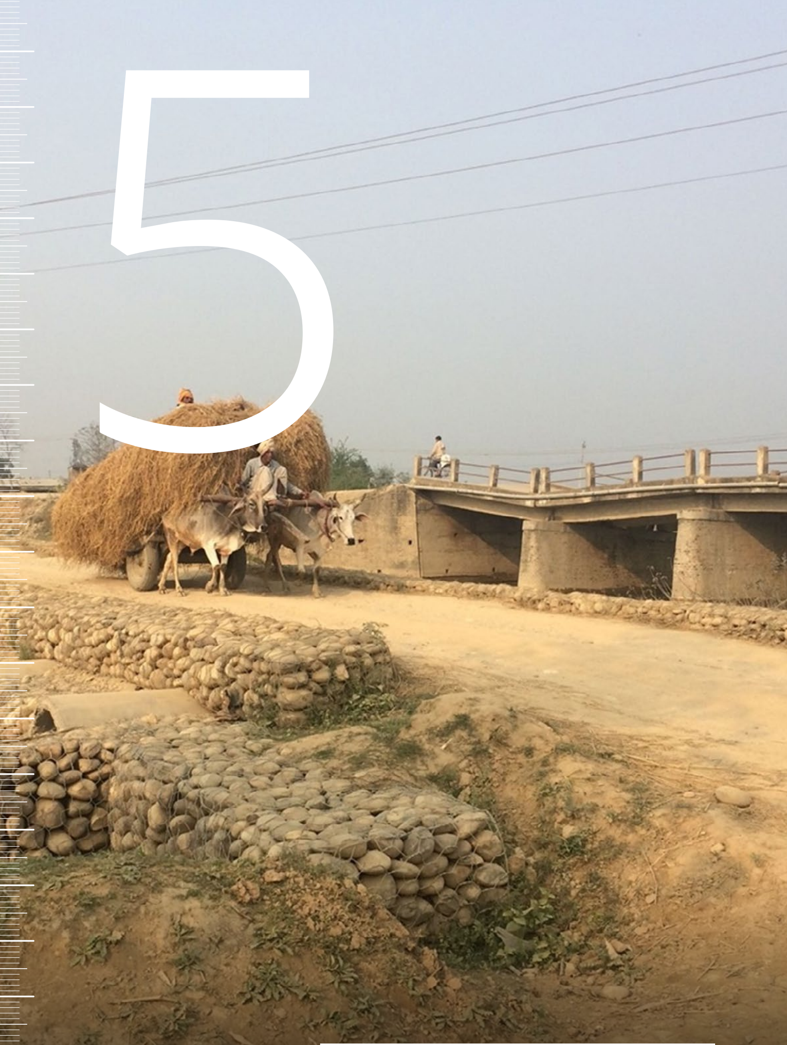
A damaged bridge alongside a newly constructed bridge in the Karnali River Basin, 2015. © Karen MacClune
