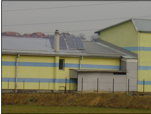
Solar panels installed on an industrial building.
